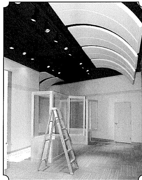
The Ojibwe Gallery remains empty until HVAC issues are fine-tuned and resolved and humidity levels can be guaranteed not to fluctuate.
